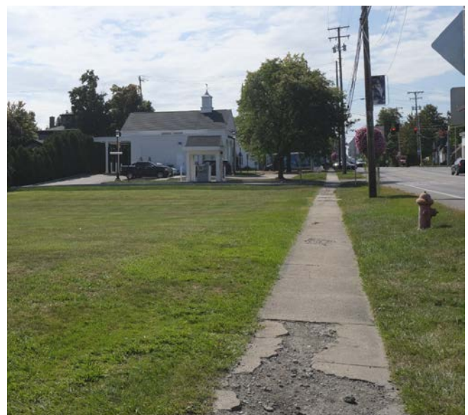
IMAGE 2-4: SR44 Sidewalk Conditions
